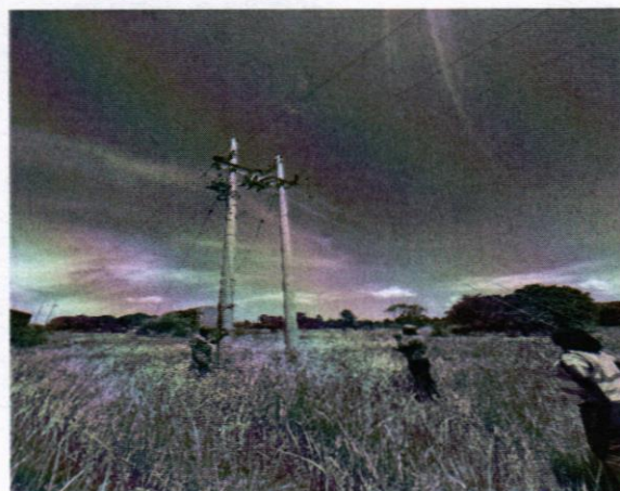
Testing of functionality of one of the installed load break switches in Baringa village, Yumbe district.
