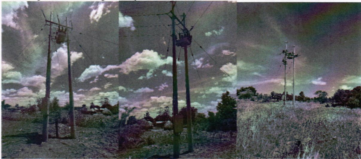
Some of the commissioned switch gears already functioning in the Wandí – Yumbe stretch.
