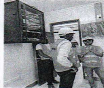
ICT Control Room
