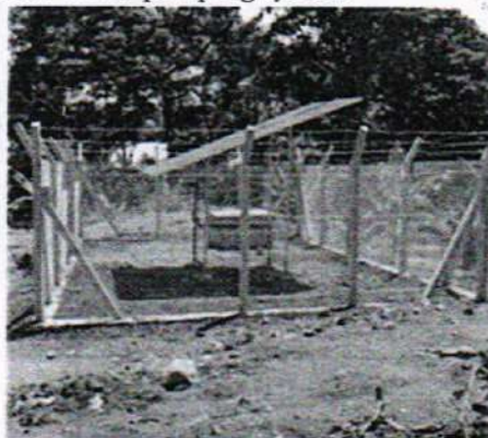
Solar water pumping system
