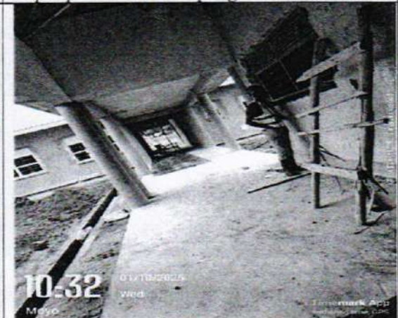
Member not aligned and has a gap
