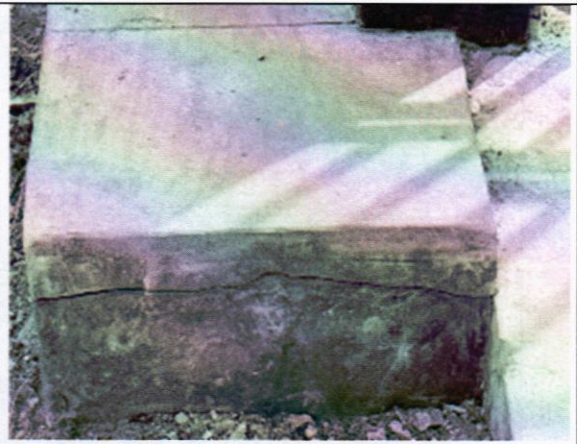
Cracked splash apron
