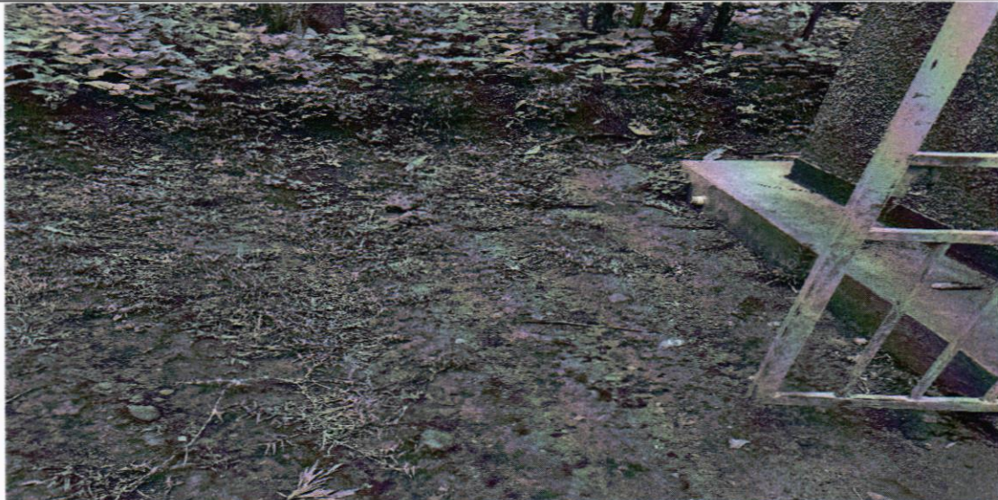
The photograph above shows the 5-stance VIP latrine at Elgon Primary School. Physical verification established that no pipe had been provided to direct drainage water to the soak pit, as indicated in the image above.
