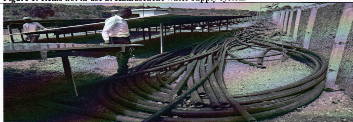
Figure 1: Items not in use at Kamusenene water supply system
