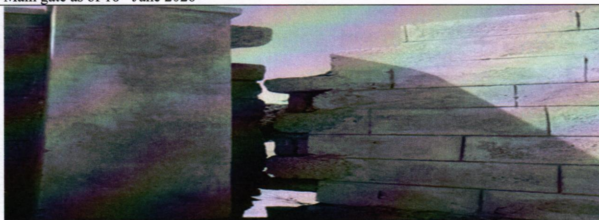
Incomplete wall fence as of 27 th November 2025
