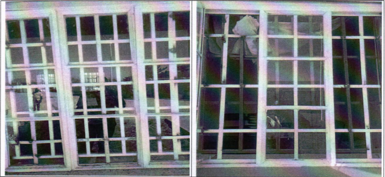
Some windows were not fully painted as of 27 th November 2025
