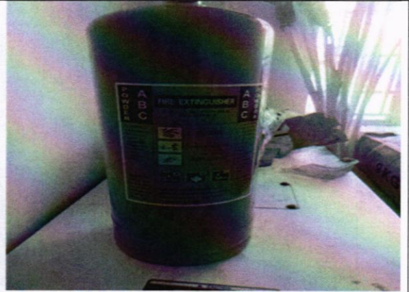
Fire extinguishers delivered but not yet installed by the contractor and not in use
