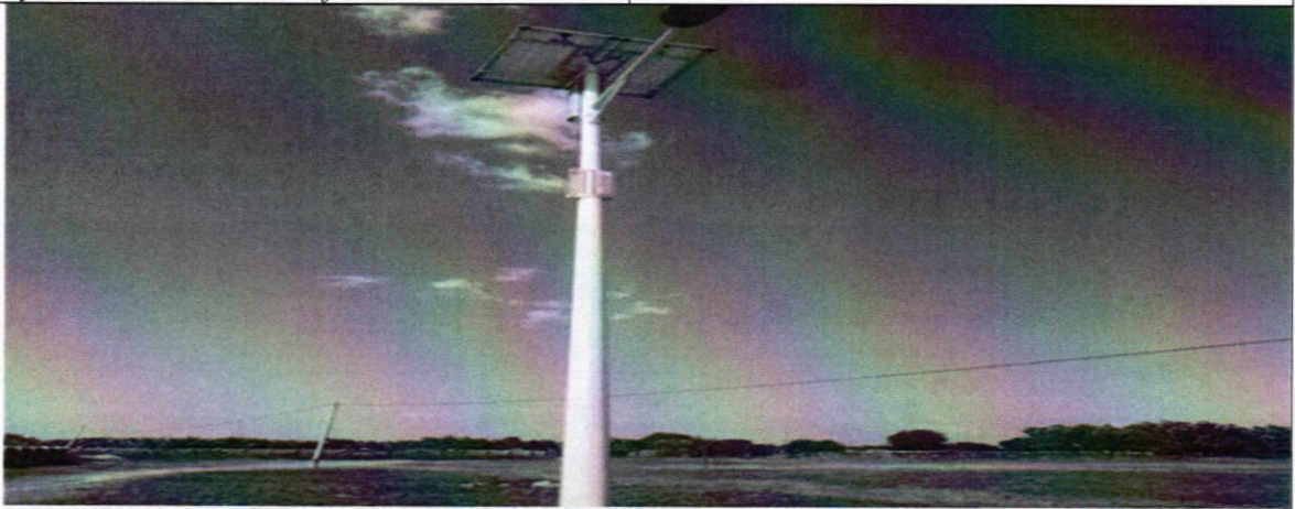
Solar lights and panels installed at Kagwara Seed Secondary School
