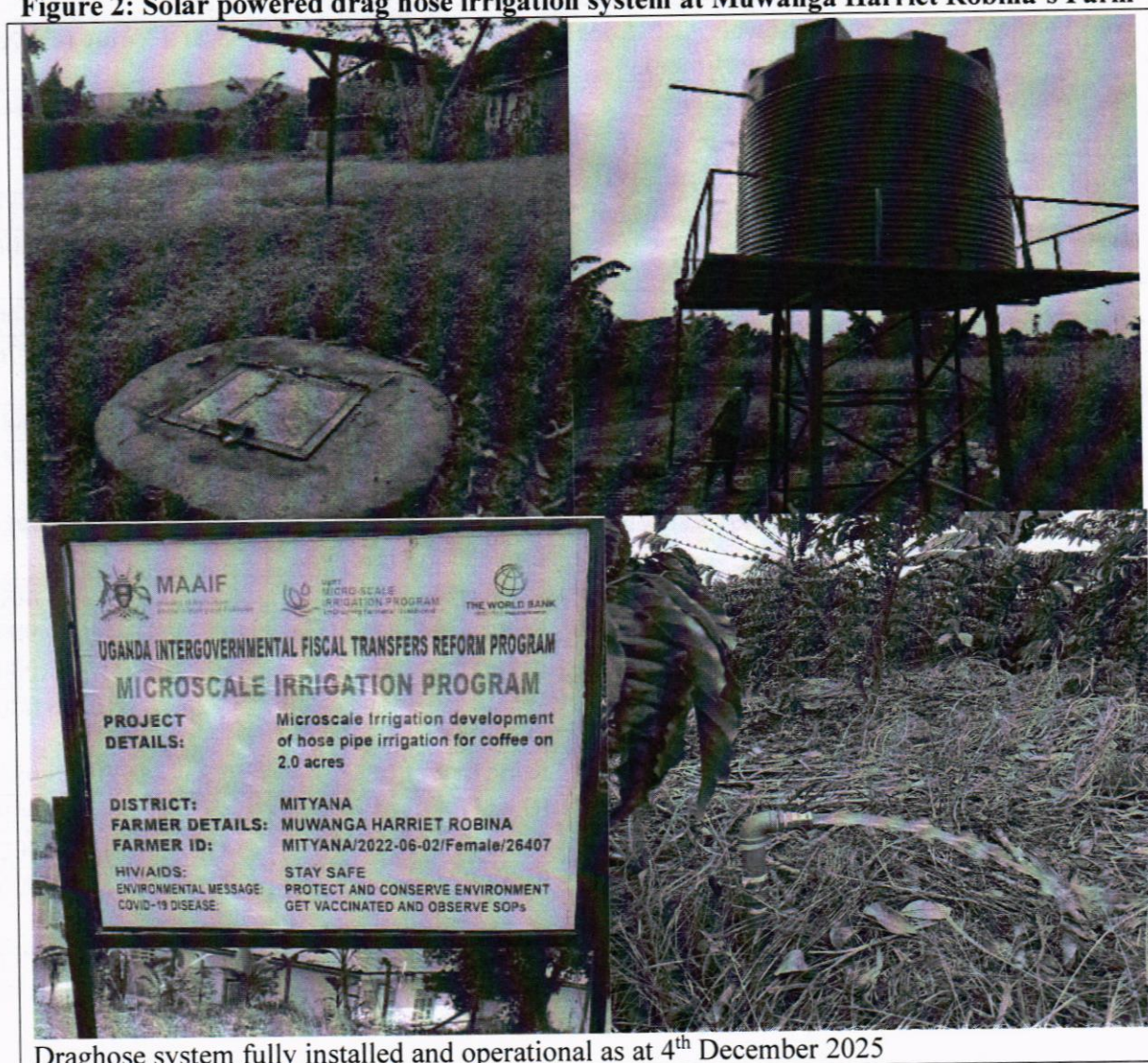
Figure 2: Solar powered drag hose irrigation system at Muwanga Harriet Robina's Farm
