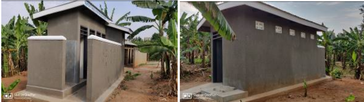
The front and rear sections of the Toilet. Picture taken on 15 th August 2019.
