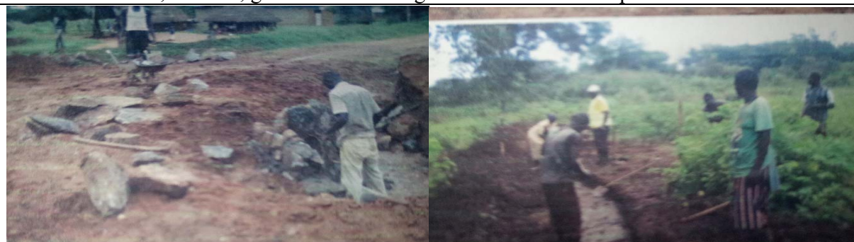
Road gang members carrying out periodic road maintenance without wearing any protective gear
