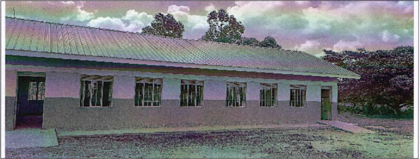
A two classroom block at Kamwalo Primary School with a leaking roof
