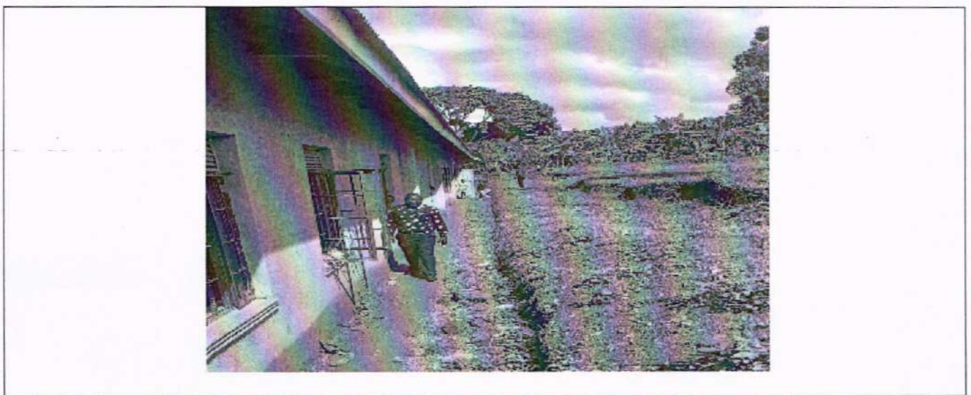
The behind veranda at Mpanga Primary School being covered by soils due to soil erosion
