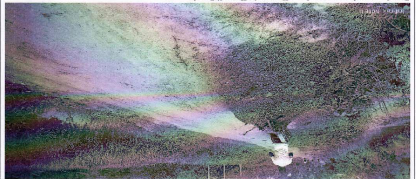
Poorly spread murrum along Kassanda Kamuli Road
