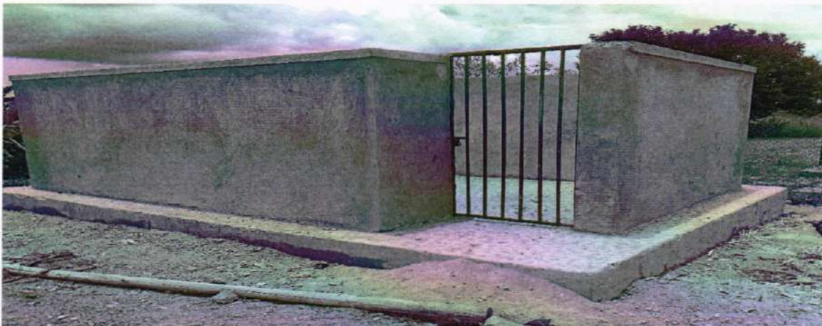
The Medical pit was incomplete due to insufficient funding and there was lid cover missing
