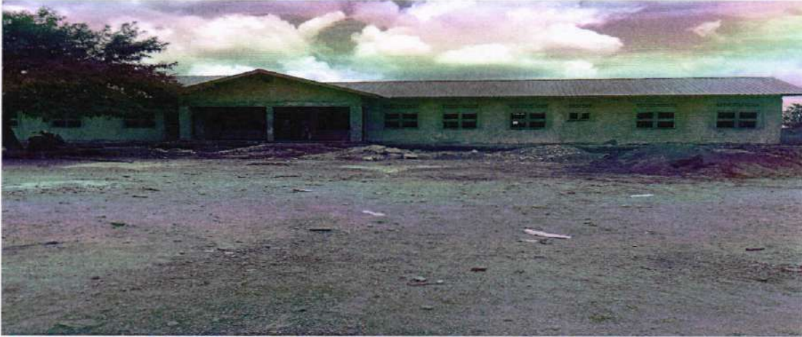
The Maternity ward was incomplete and had been abandoned due to funding shortfalls
