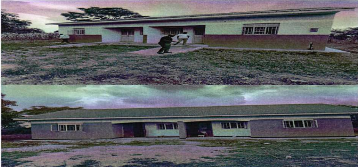
Figure 1- Status of construction of 2 staff houses at Kaliro TC HCII and Kisinda HCII.
