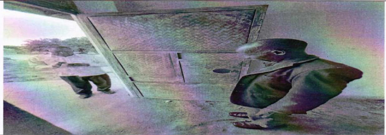
Unpainted doors which are likely to rust
