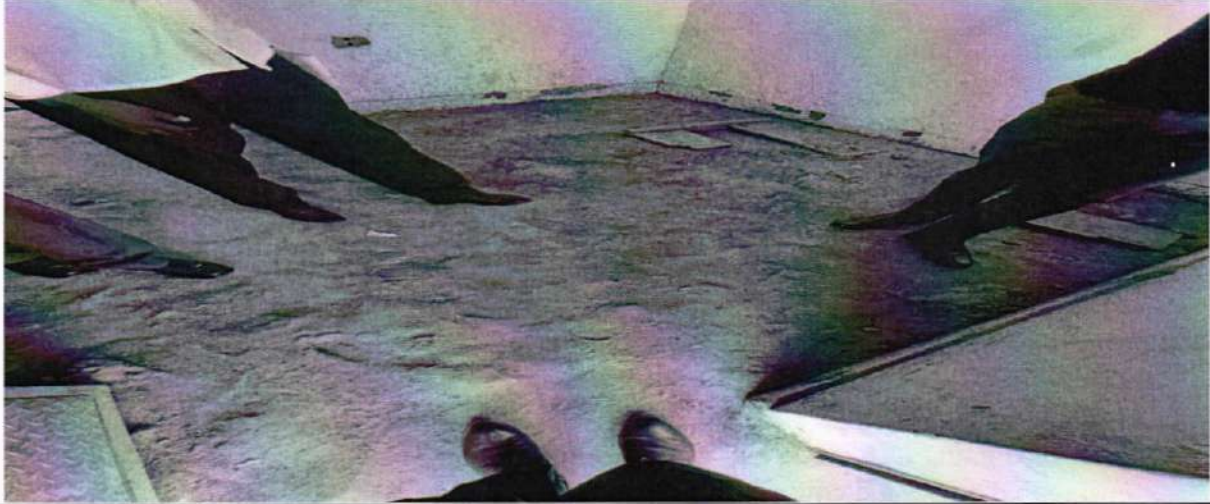
Incomplete floor in the Head Master's Office
