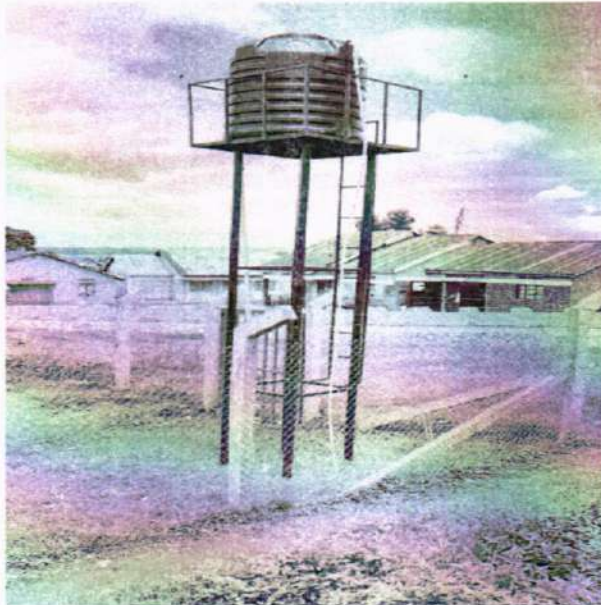
Below: The water tank
