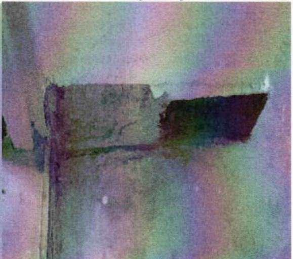
Poor workmanship on the outside skirting
