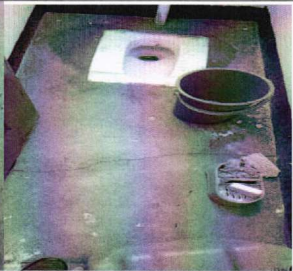
Visible cracks on the floor of the bathroom
