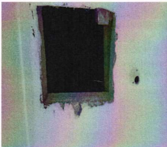
Poor workmanship works around the ceiling hole
