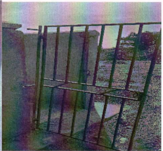
Poorly installed burglar at the entrance
