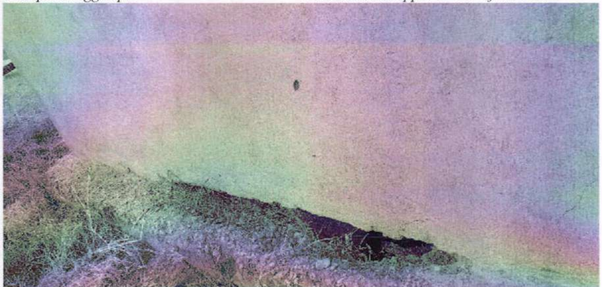
Huge crack at the wall foundation
