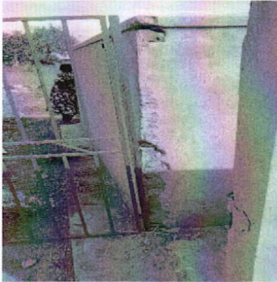
Poorly installed burglar at the entrance
