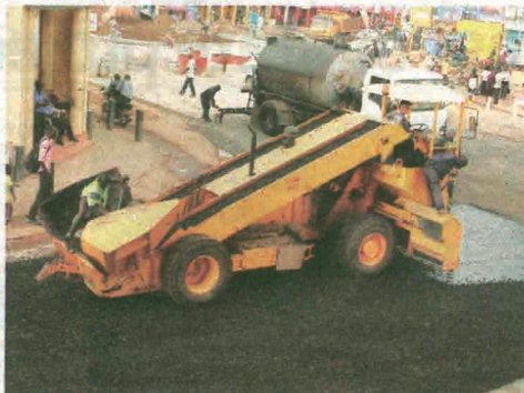
CICO construction workers working on a road section in Arua Town. Subcontracting usually happens in complex projects such as construction. PHOTO BY CLEMENT ALUMA
