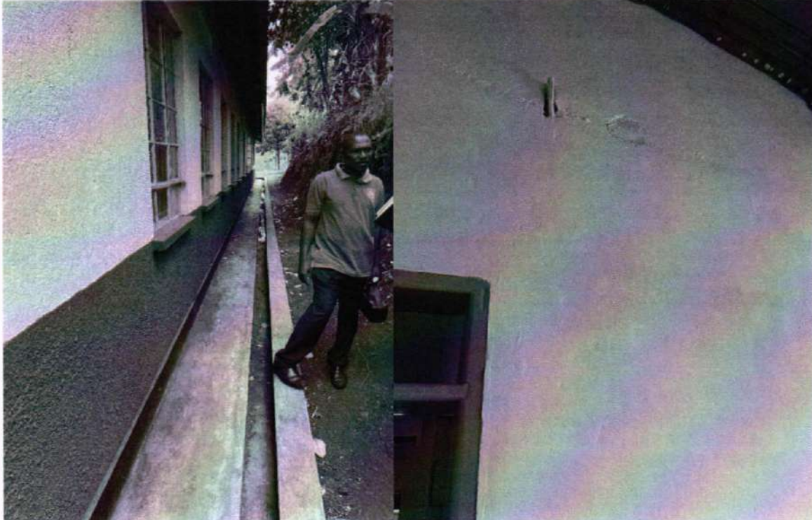
Poorly drainage around the block
