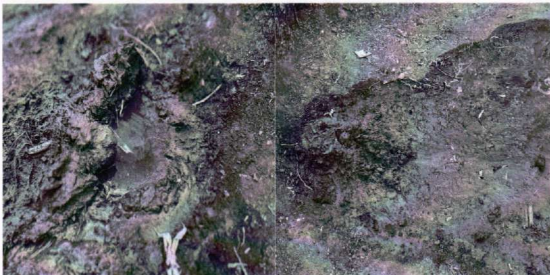
Uncontrolled water leakage due to compromised pipe integrity causing inefficiencies in the system.
