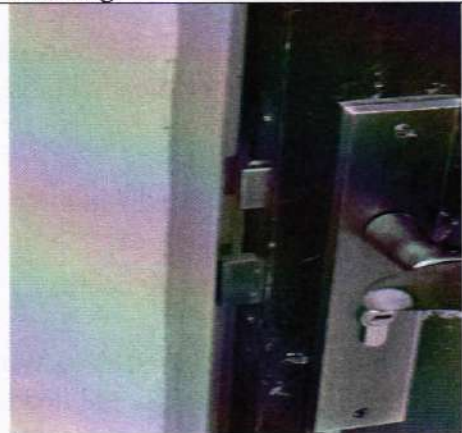
Unlockable and defective door lock in the interior of one of the houses.
