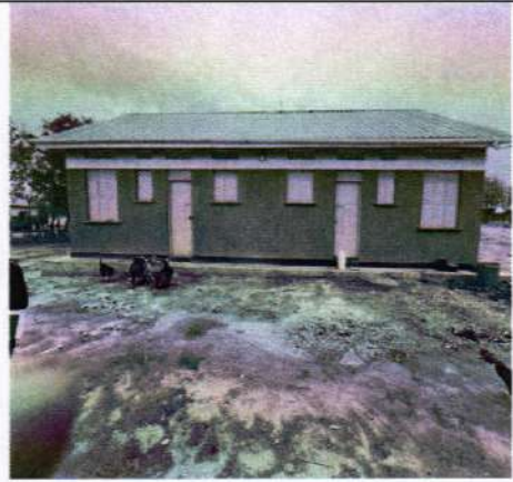
Back view of staff house showing the lightning arrester without earthing
