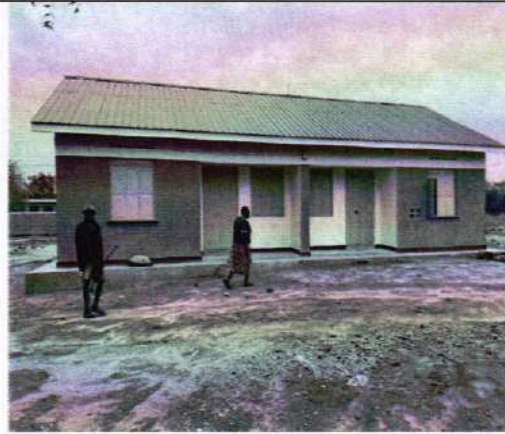
Front view of staff house without a ramp to ease access.
