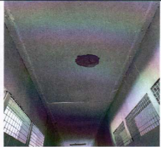
Wooden ceiling corridor with a central water stain or damp patch visible on one of the ceiling panels, indicating a possible roof leakage or water infiltration.
