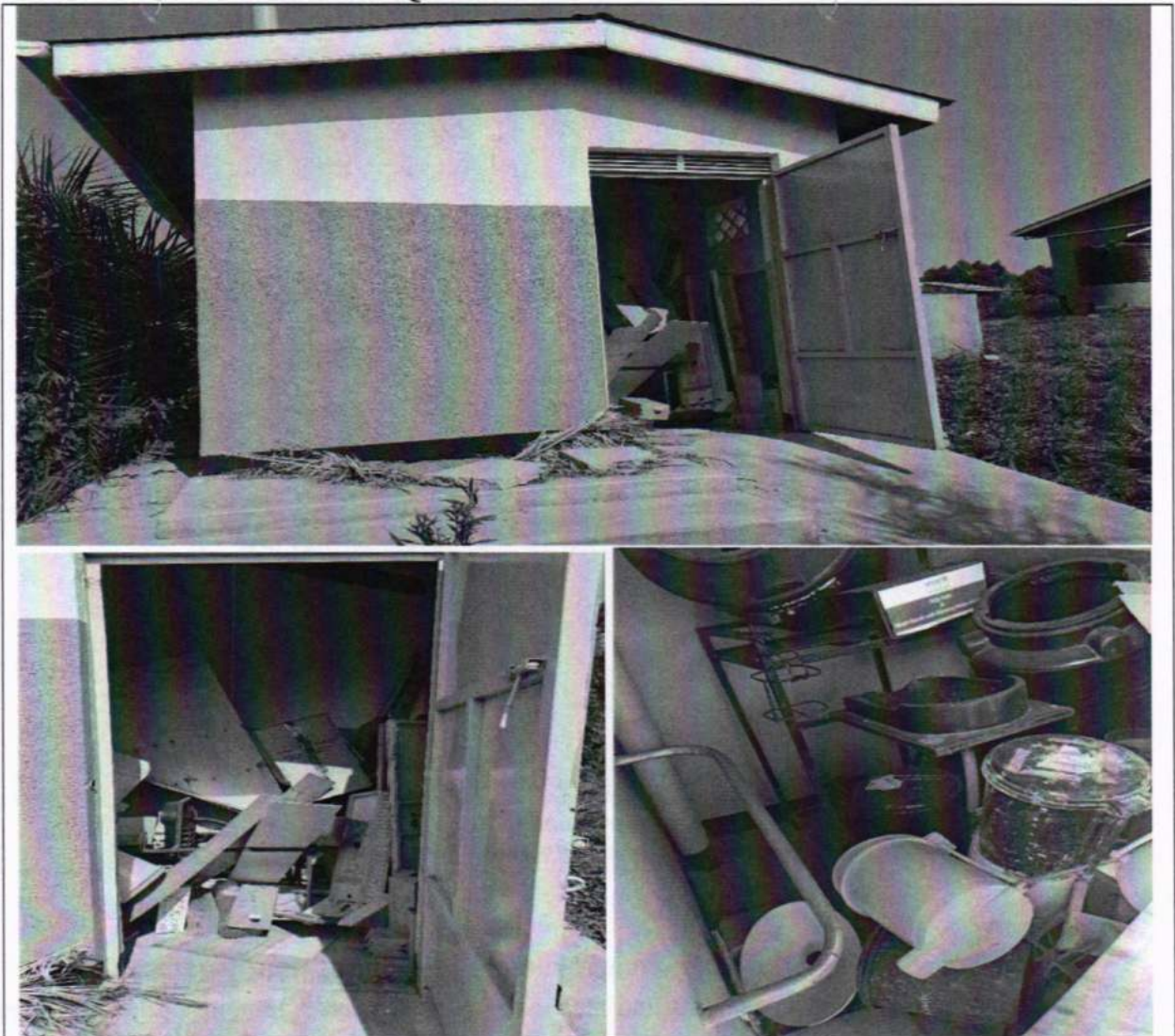
Figure 4: Physical Status of the construction of 5 stance lined latrine at Lucy Bisereko Health Centre II for the Staff Quarters
