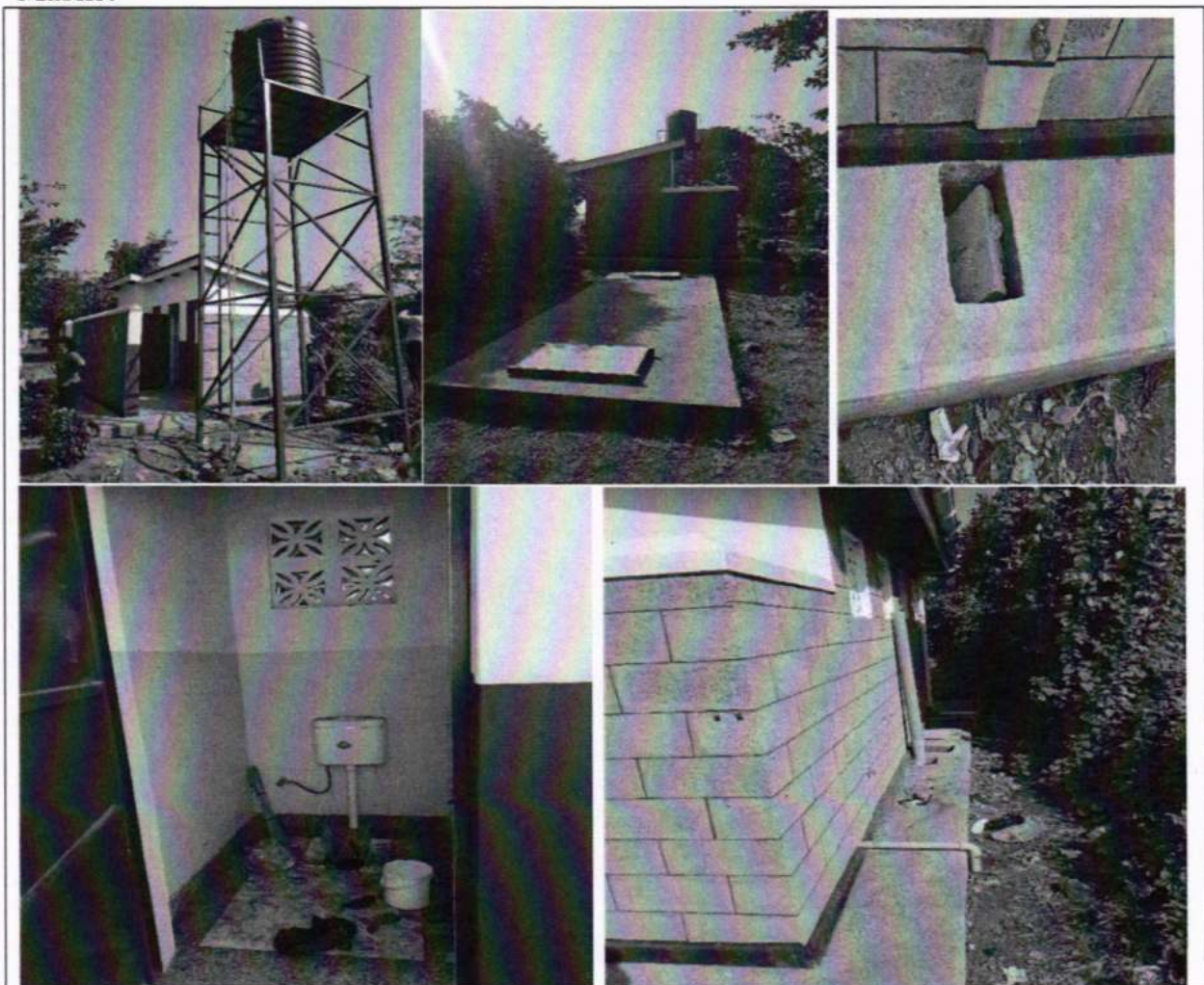
Figure 5: Physical Status of the construction of 4-stance water borne toilet at Kinogozi Market
