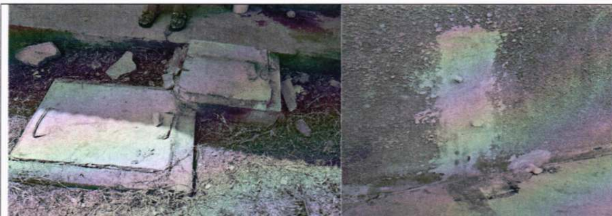
Poor finishes for Repair Works & Septic tank Construction at Wambabya HC III
