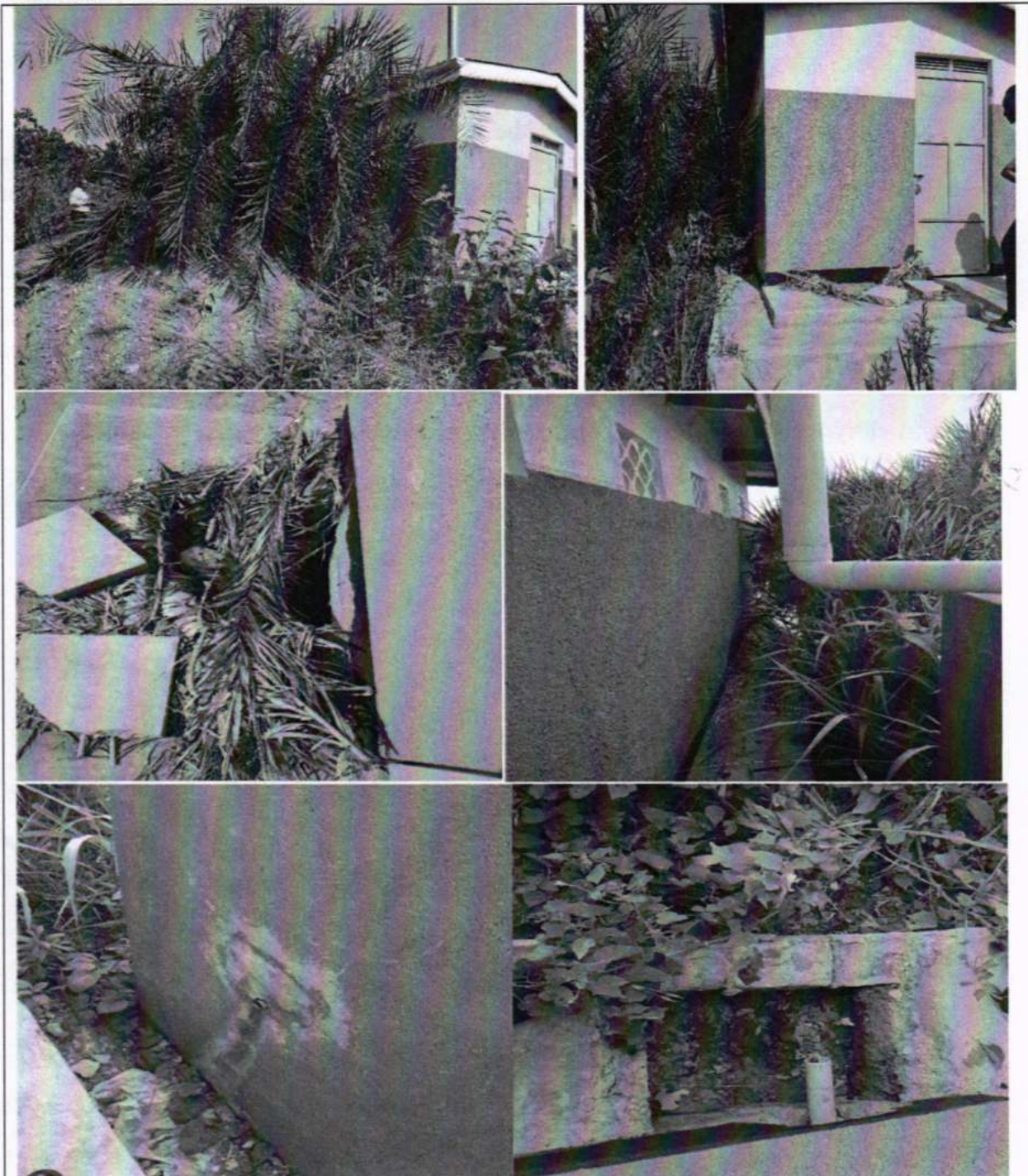
No ground levelling, incomplete plumbing works and with palm leaves as provisional cover of the manhole pit for the five Stance Lined Pit Latrine Block at Lucy Bisereko Health Centre II
