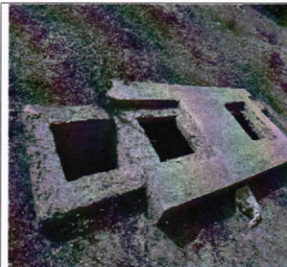
Uncovered septic tank
