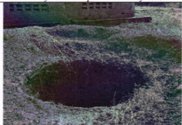
Incomplete soak pit for maternity block
