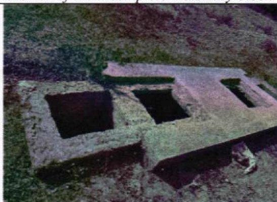
Incomplete septic tank for maternity block
