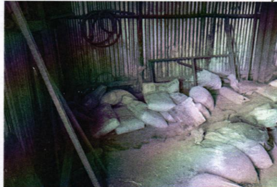
Cement stored on ground instead of a raised surface/pallets
