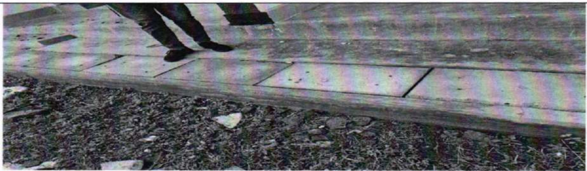
The Slabs for the storm water drainage were developing cracks and needed to be redone.
