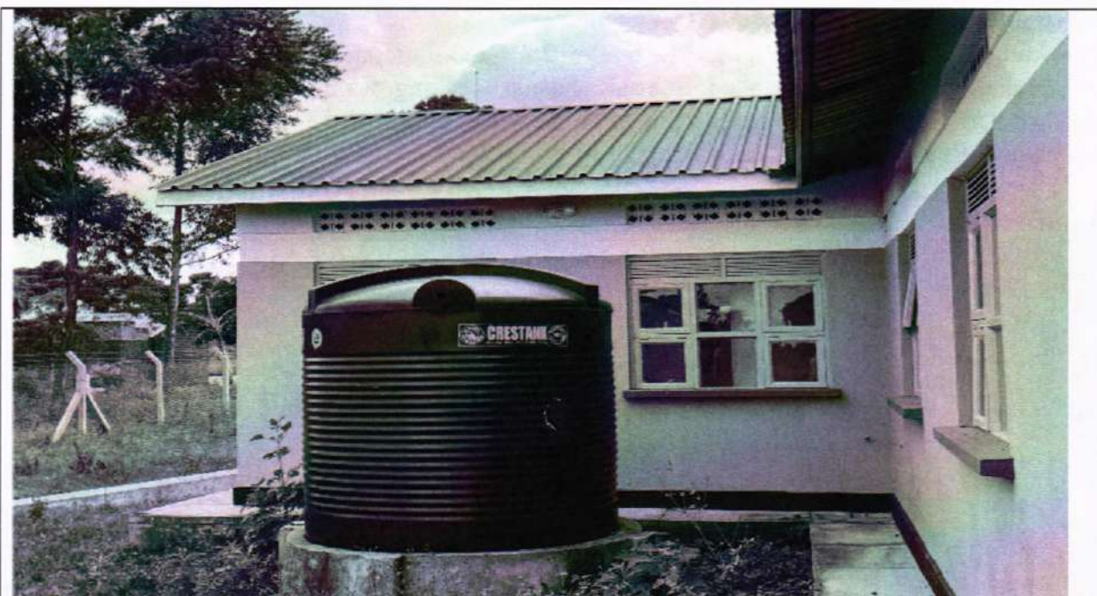
Rainwater harvesting works not done e.g. fixing of gutter and pipes
