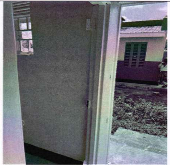
Internal doors not fitted
