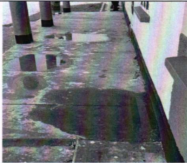
Water collected on poorly levelled floor
