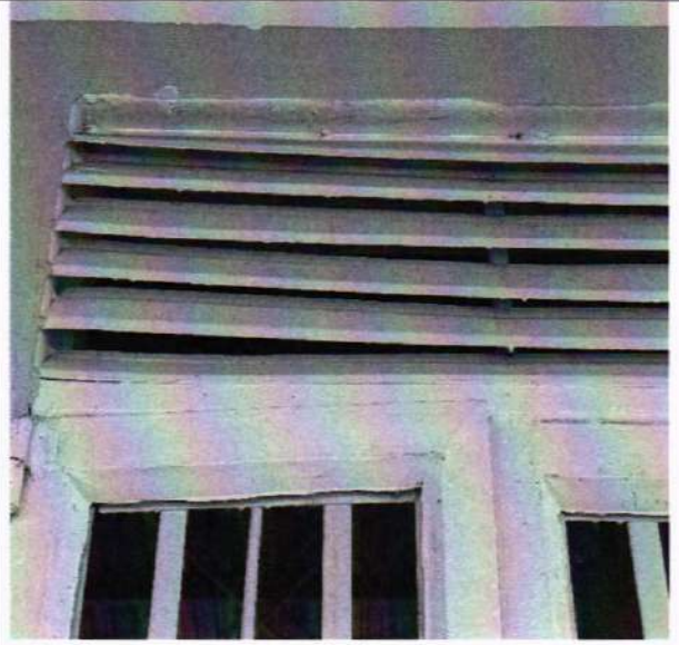
Window vents not well aligned
