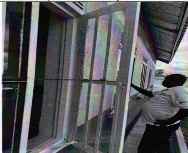
Burglar proof fixed on the window instead of fixing directly on the main window frame
