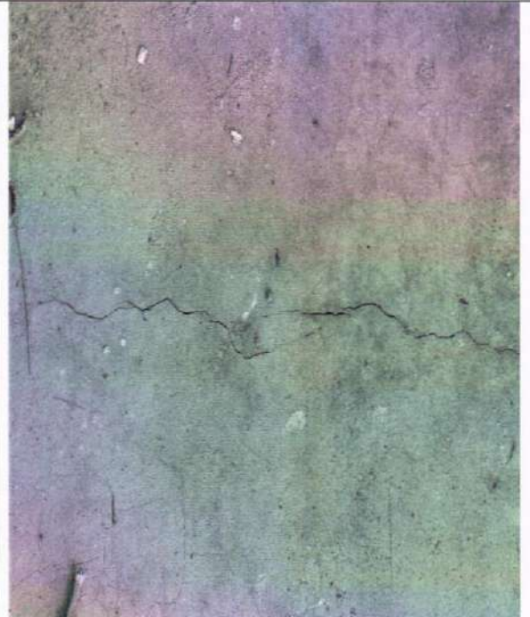
Cracks on the floor of the staff house
