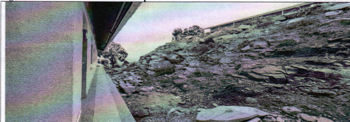
Fig 1: Shows different sections of steep embankments on the rear side of the classroom blocks
