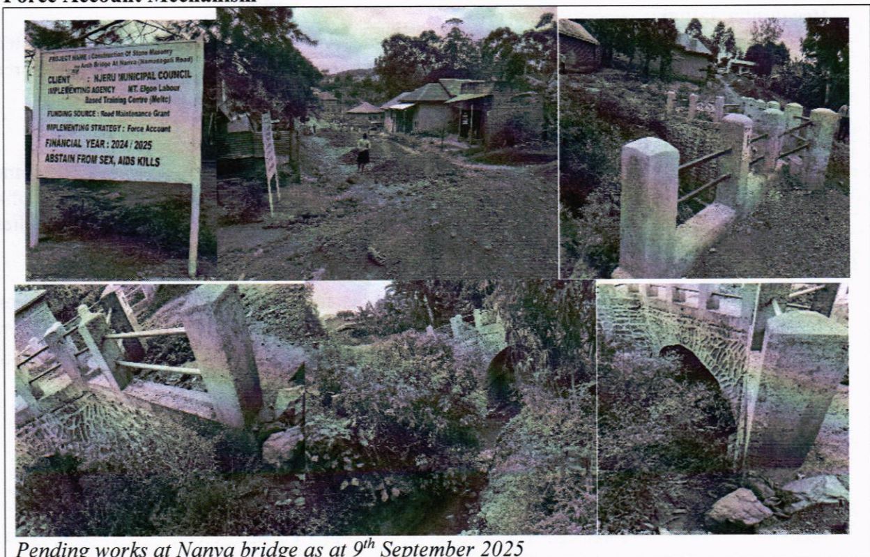
Figure 4: Construction of stone masonry arch bridge at Nanva (Namasagali Road) using Force Account Mechanism
