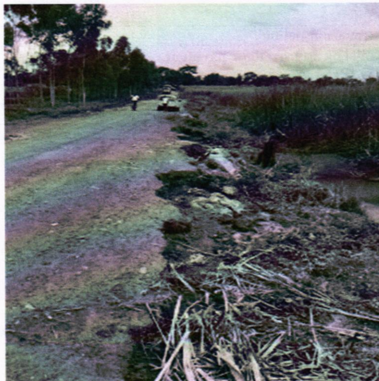
Severe damage to the road due to sugarcane trash at Kinawanswa – Kawangera swamp
