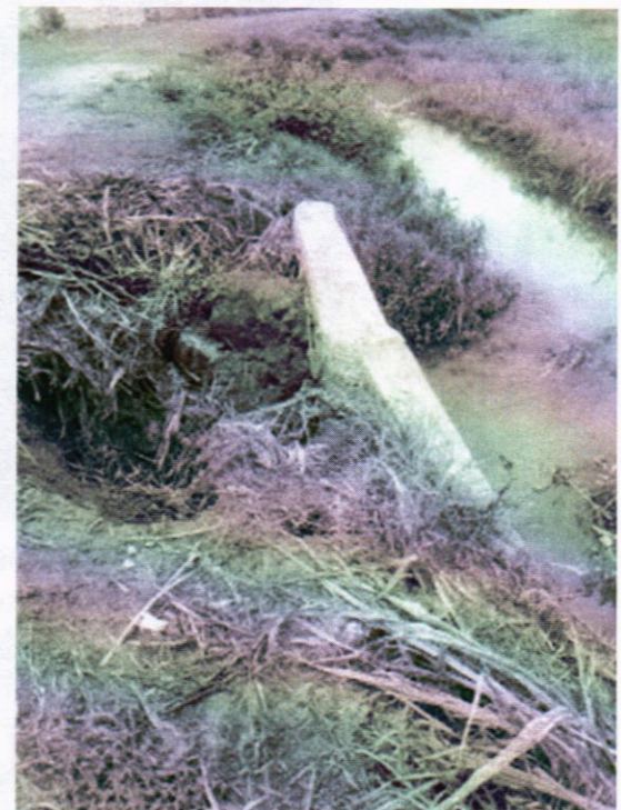
The sugarcane trash at Kinawanswa – Kawangera swamp resulting in over flow damaging the new road
