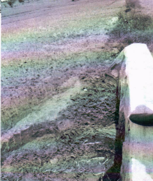
Rice growing activity up to the road side channel and culvert at Irenzi-Kabugo swamp resulting into silt blockage of water flow
