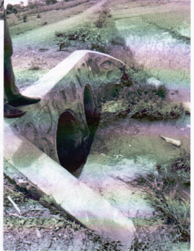
Rice field causing stagnant water likely to weaken the road foundation at Irenzi – Kabugo swamp
