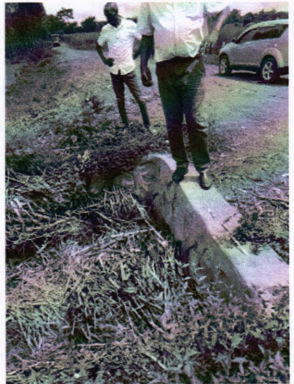
Another culvert at Kinawanswa – Kawangera swamp blocked by trash
