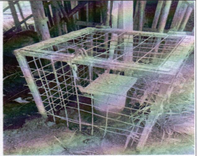
Borehole at Laropi WTP
