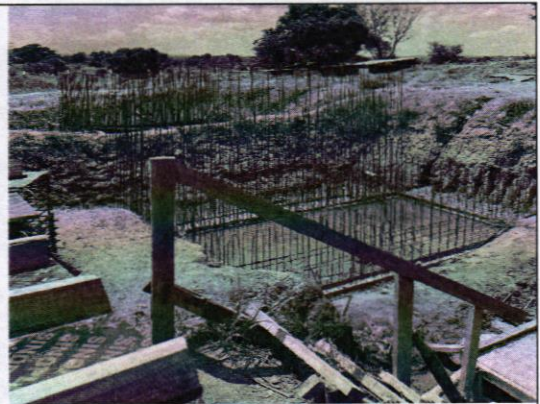
Filtration Tank at Gwere WTP
