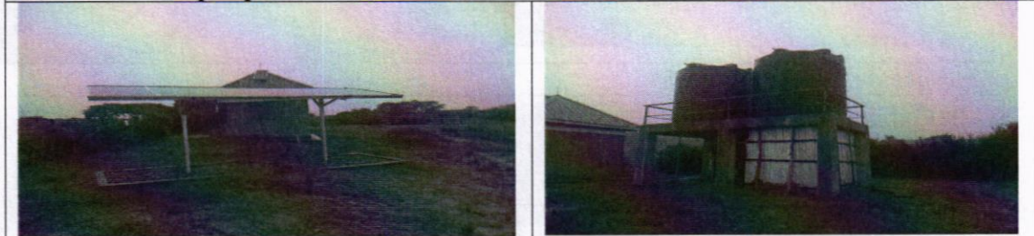
Solar pannel system and two 10,000 litre tanks
