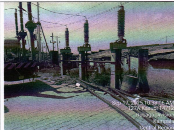
132kV feeder to the main transformer
