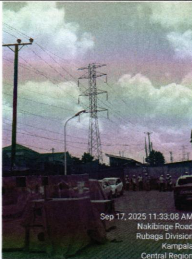
One of the towers of Kampala North, Mutundwe, 132 kV transmission line
