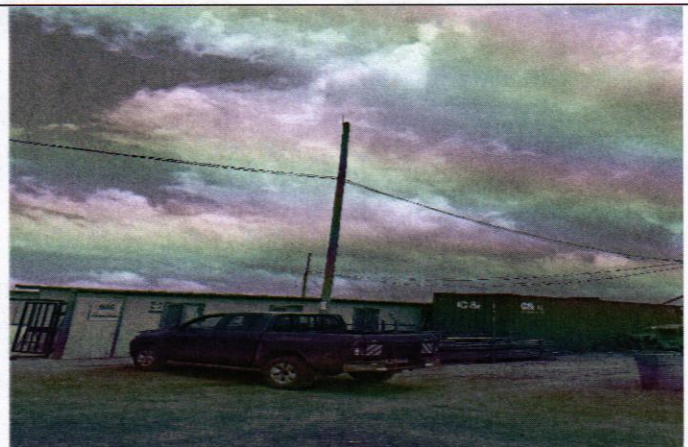
Existing Low voltage network supplying offices, campsite and all infrastructure around the site
