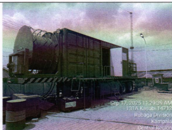
The general view of MV Trailer 2, which holds the auxiliary transformer, voltage monitoring, and control units (steps voltage to 33kV and 11kV)
