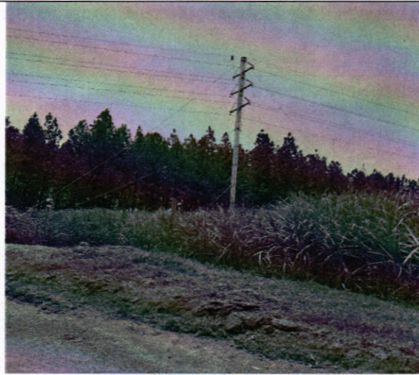
Emergency restoration tower wind stays footprint encroaching on the road and at risk of being knocked
