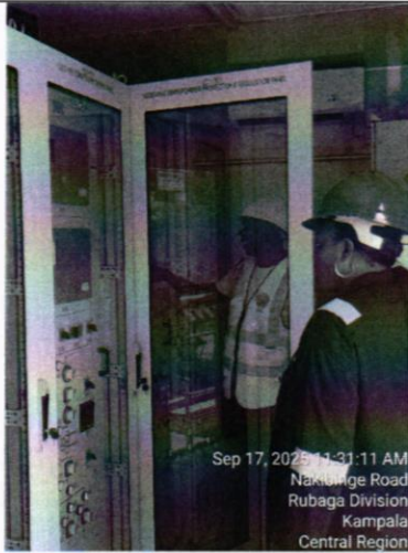
Voltage monitoring and control/protection cabinet in Trailer 2
