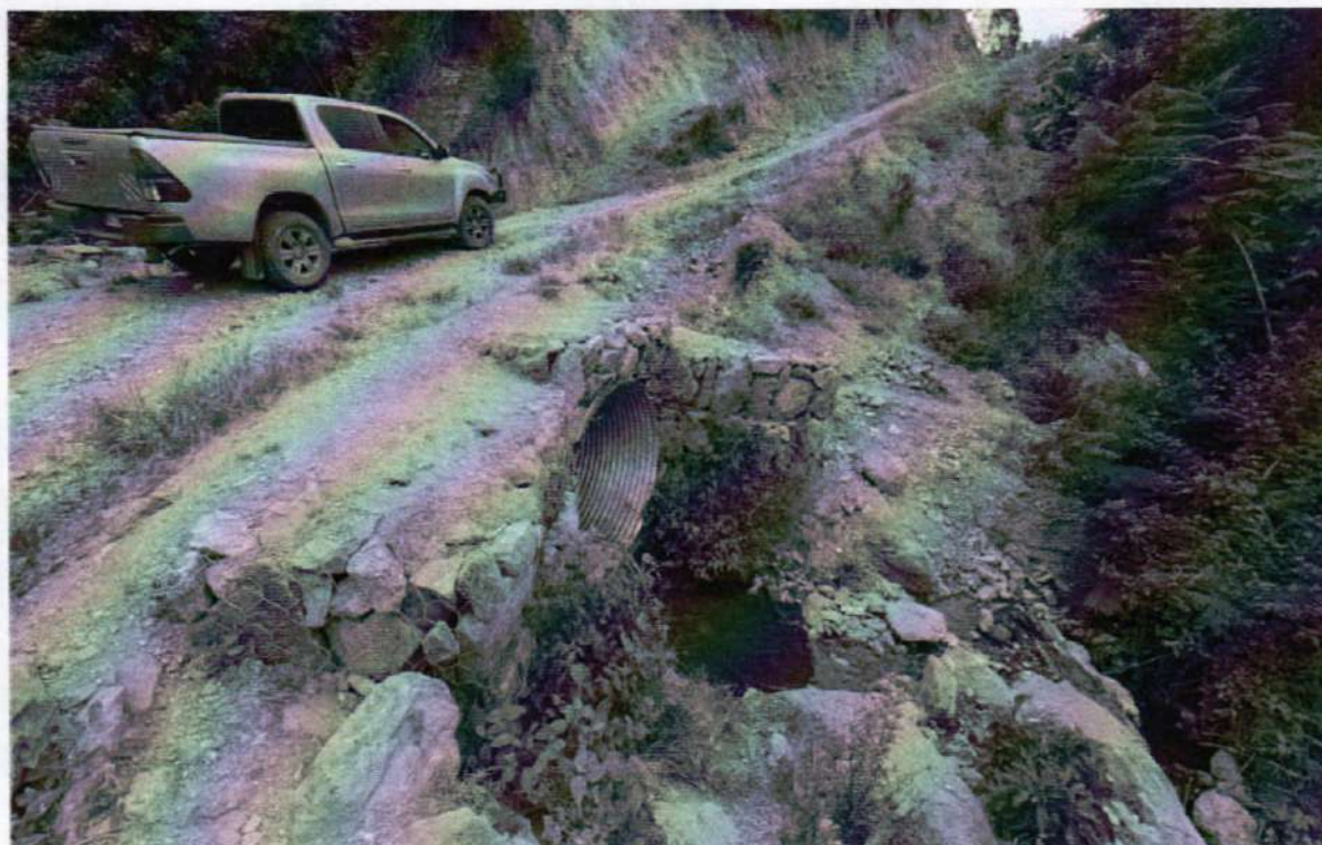
Image 15 shows an opened section of Burondo Road
