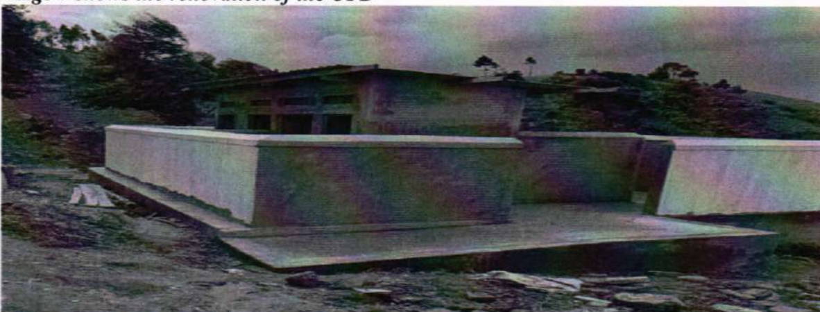
Image 8 shows the 5 stance VIP Latrine
