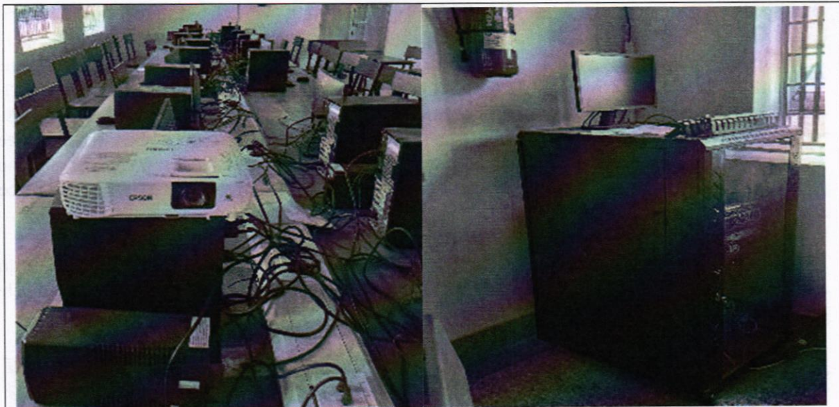
ICT equipment at Nsambya Seed Secondary school not engraved as at 31 st March 2026
