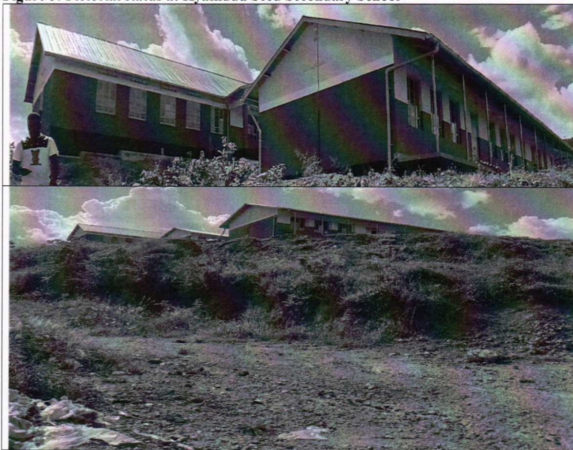
Back View of the School facilities(Classroom Blocks) that require stone pitching and retaining wall -27 th March 2026
