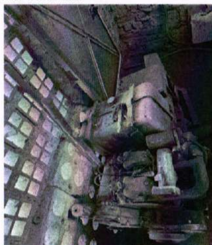
Non-functional generator in the
