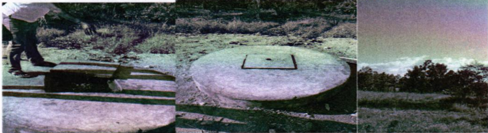
Complete water source not connected to the tank
