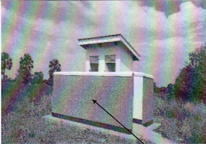
The two stance VIP latrine was not labeled.
