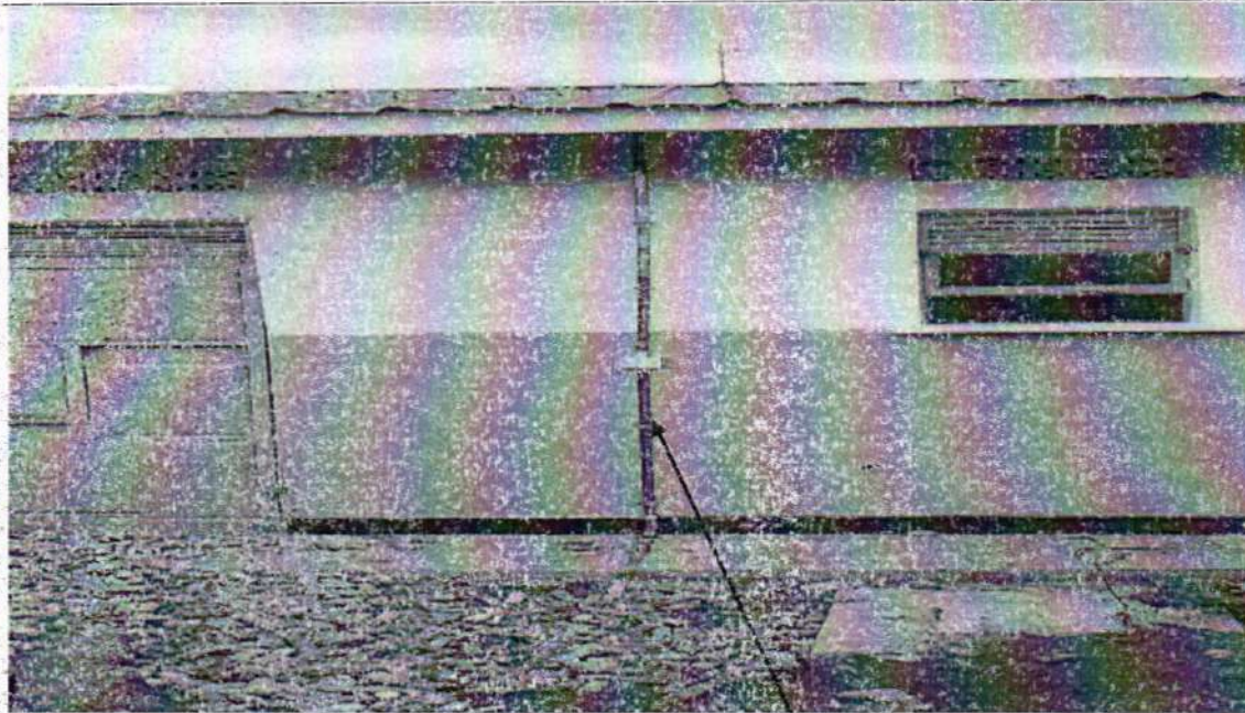
The copper wire of the lightning arrester was left exposed
