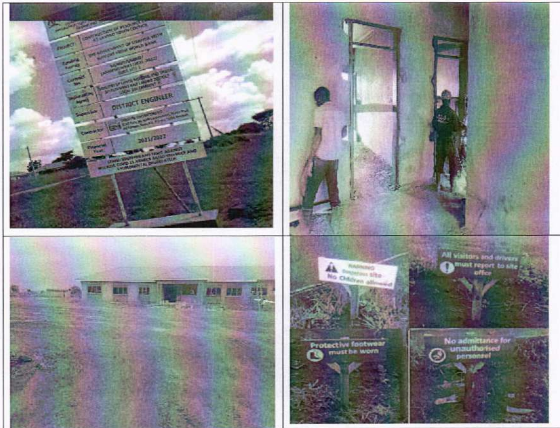
Figure 3 shows the status of the contract for construction of the resource centre after the audit field exercise
