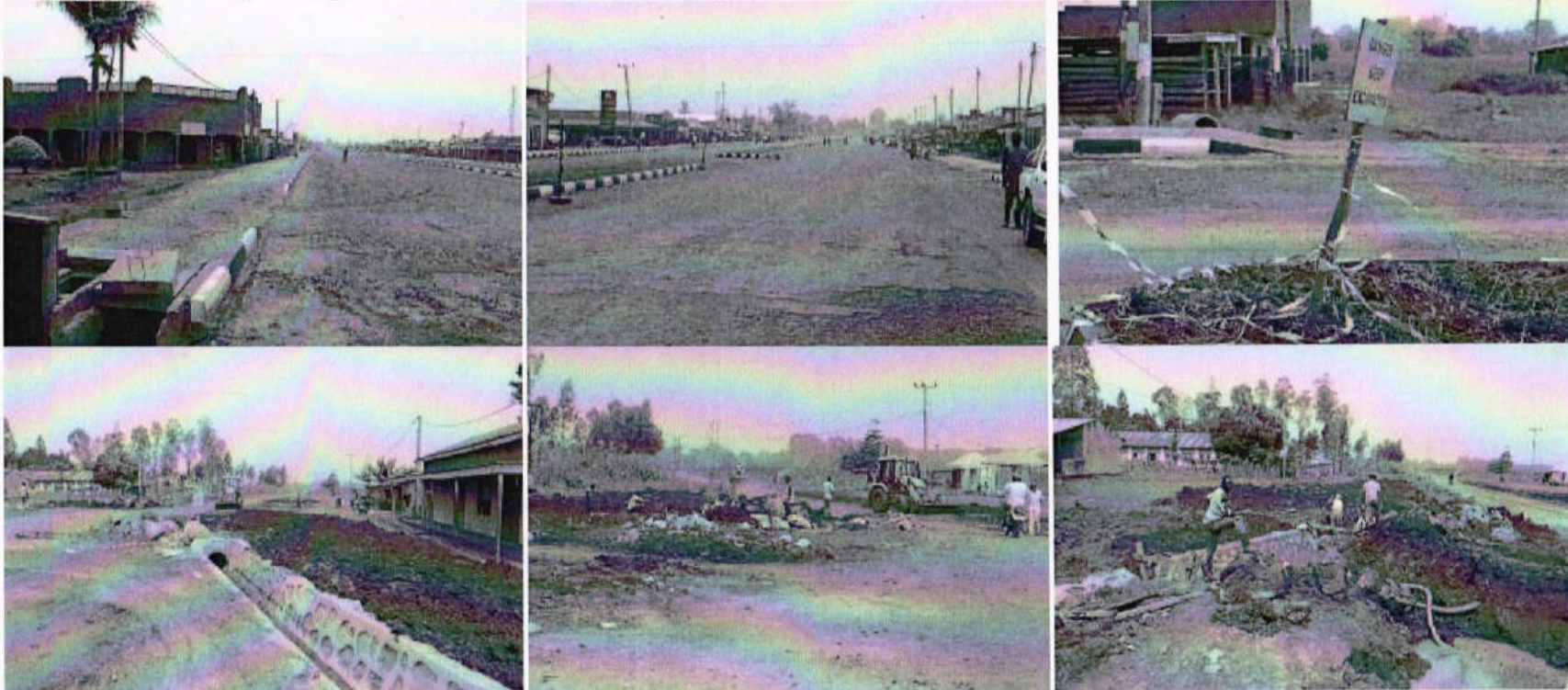
Photographs showing incomplete construction works and workers without PPEs on Chegere Road.
