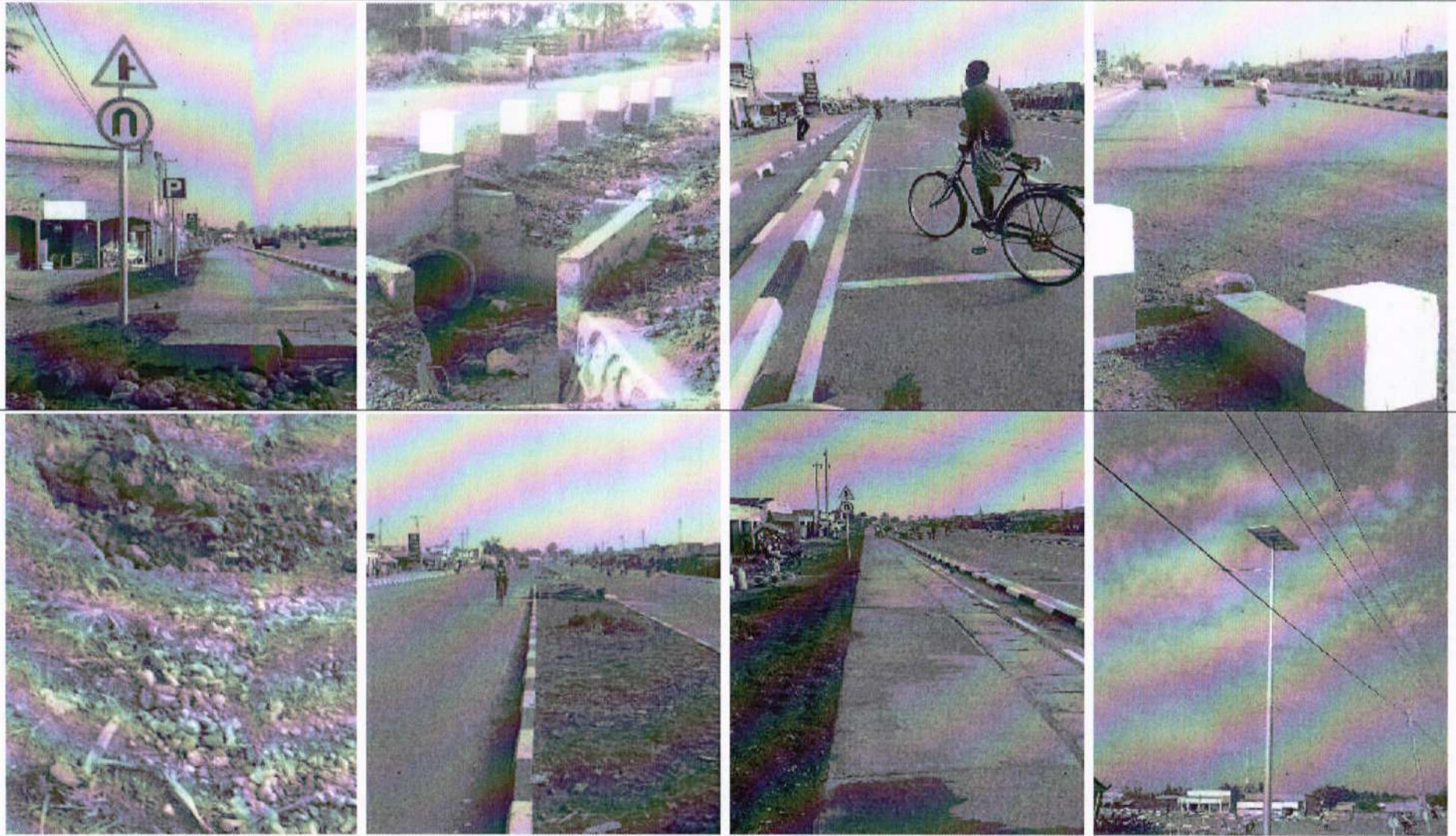
Ancillary road works including street tree planting, road marking and road signage have begun.
