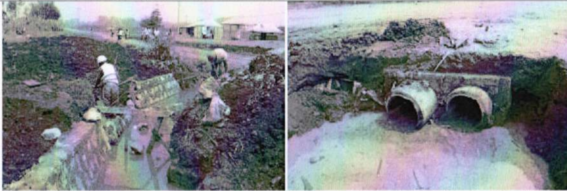
Photographs showing water filled excavated drainage channels on Chegere Road. As seen in the photos it's very risky to cross over the drainage channels, the stagnant water is a breeding ground for mosquitoes.
