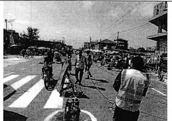
Contractor's workers on site without appropriate PPEs
