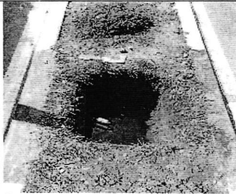
Dangerous uncovered holes dug for street light installation
