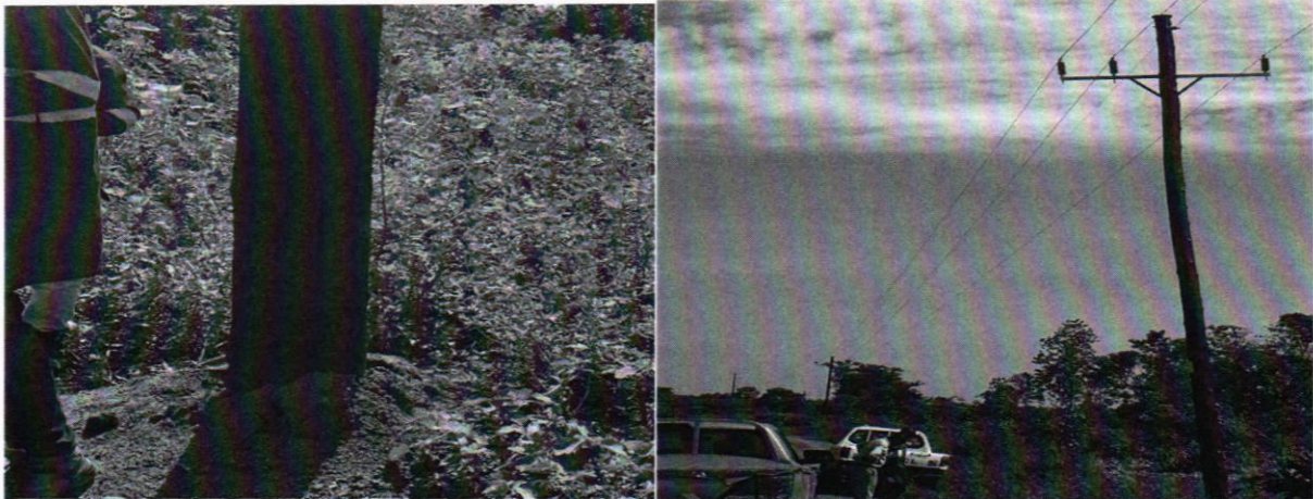
Figure 1: Pole on the verge of falling
