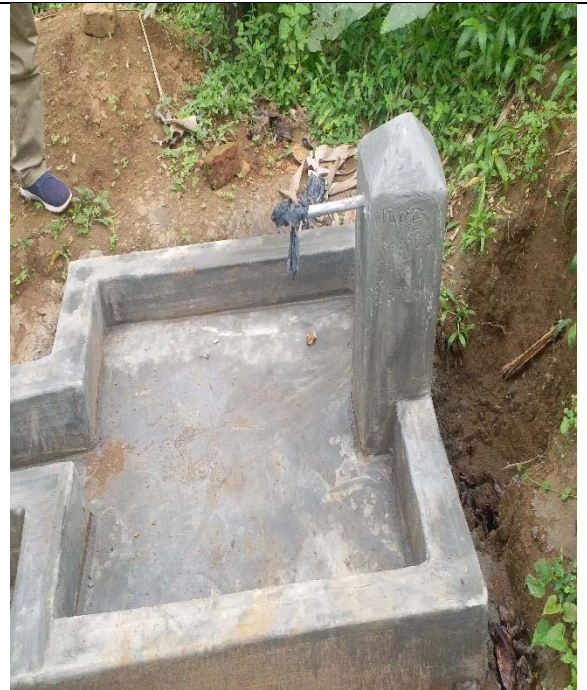
Captioned above is a sample of the tap stands installed at Namulwe S/C, Bubiita S/C and Nanyinza S/C. These are pending connection
