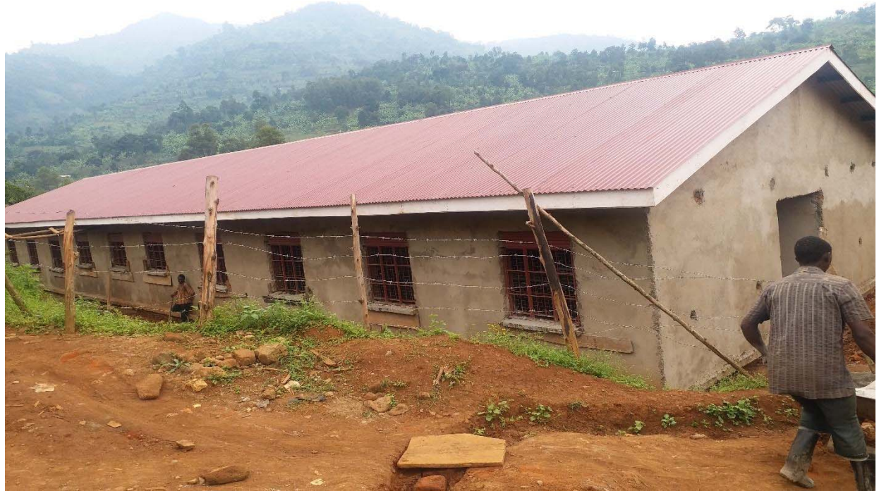
Captioned above is the ICT Laboratory block with library. Works were at interior plastering
