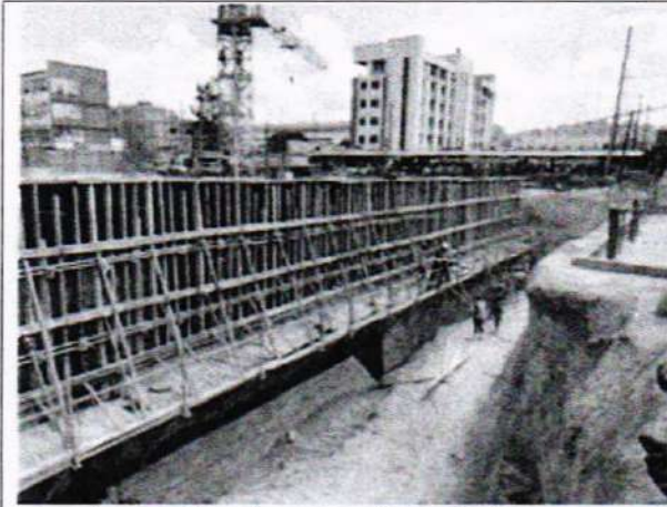
Ongoing works of construction of a large retaining wall. The wall structure is supported by scaffolding and wooden formwork.
