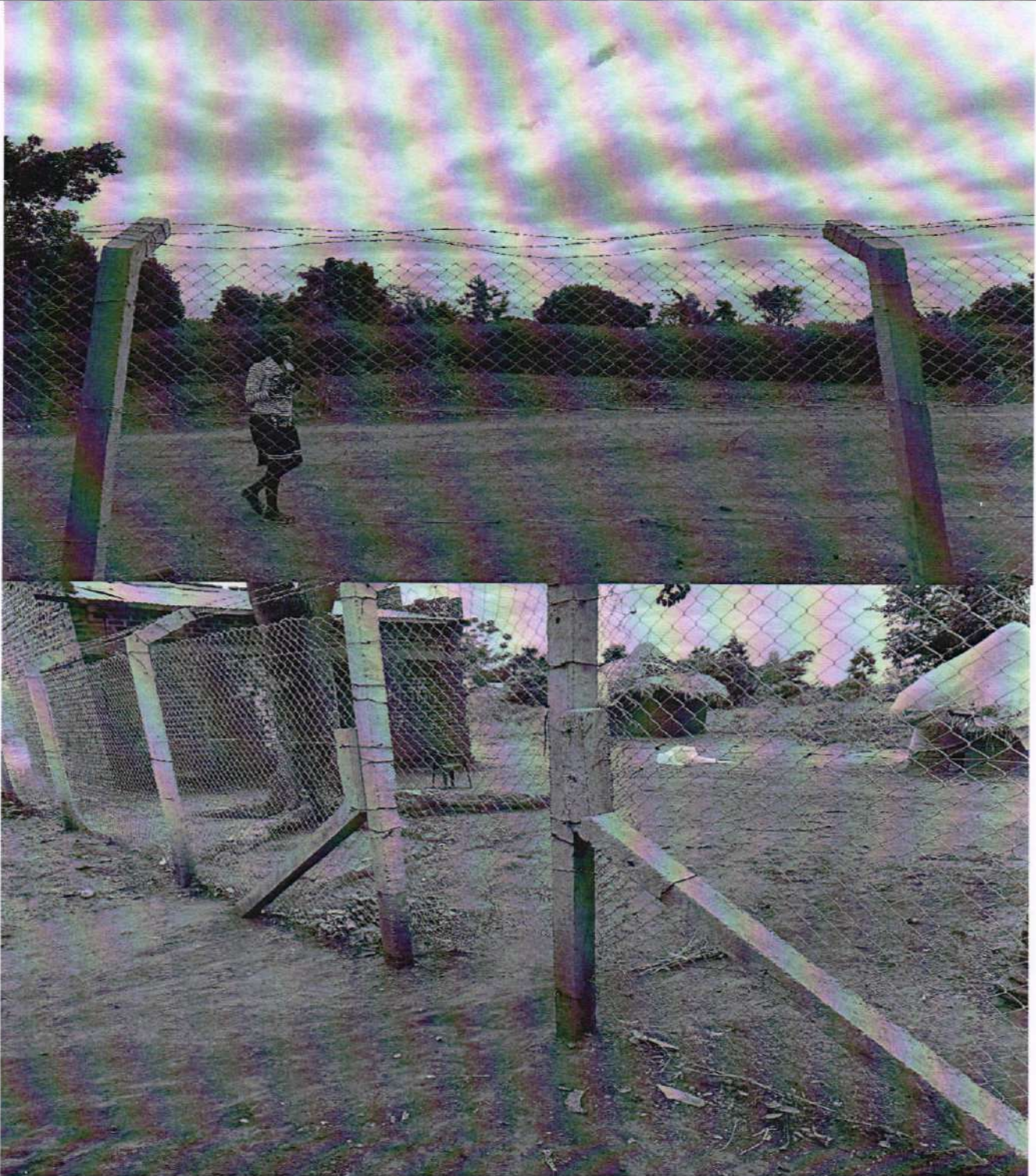
The chain wires at the top had not been stretched properly Part of the fence had been vandalised
