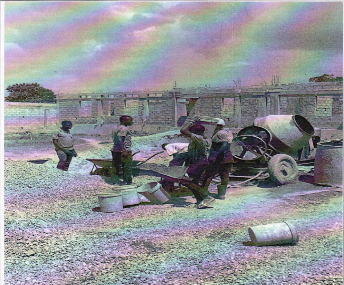
Site personnel working with no personal protective equipment
