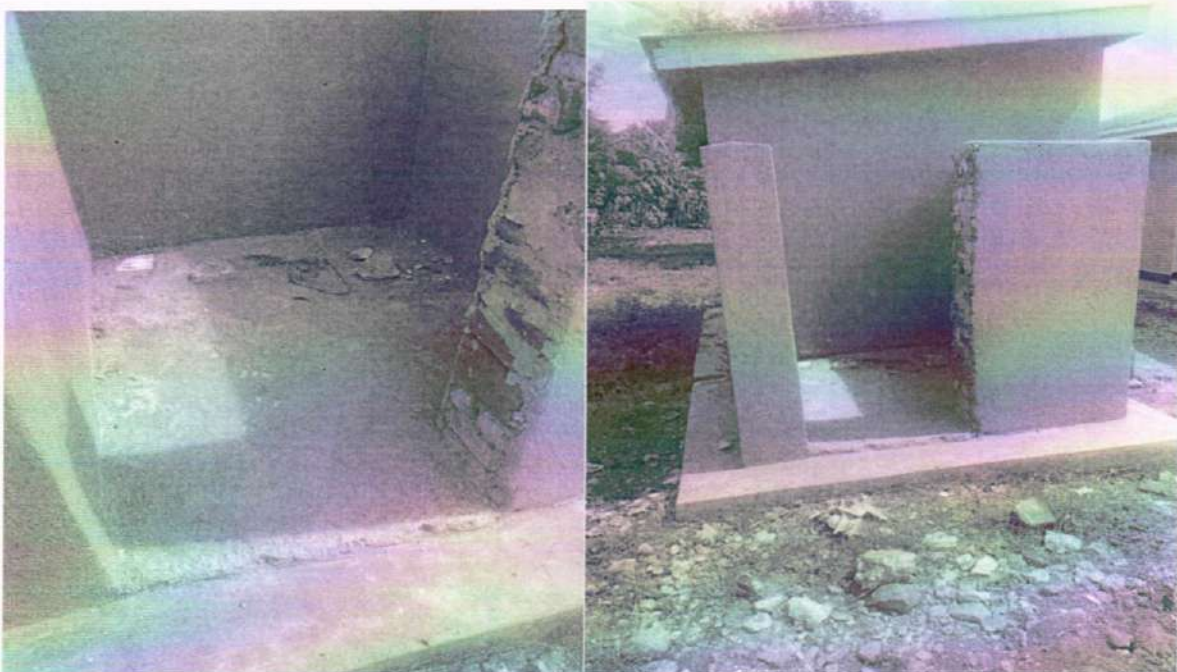
Unfinished floor of the bathroom
