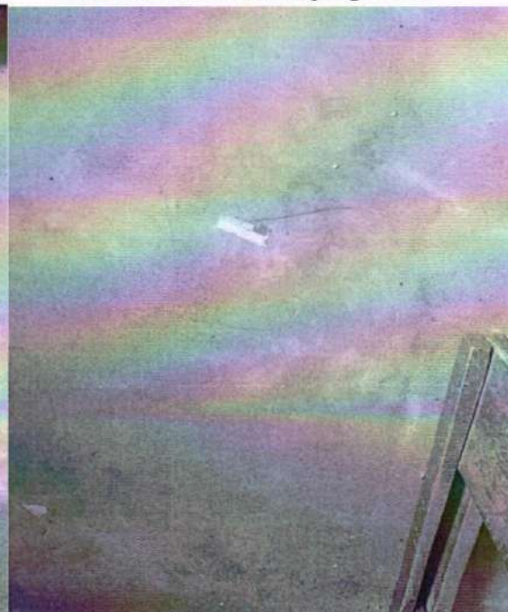
Developing cracks on Classroom floor
