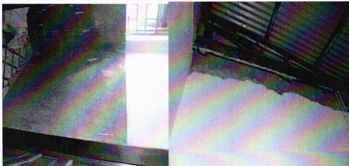
Poorly designed bathroom of small size (83cm by 100cm). Poorly completed. The walls were not fully plastered
