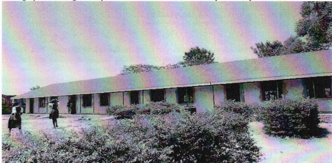
Photographs showing incomplete construction works of Dranya Primary School
