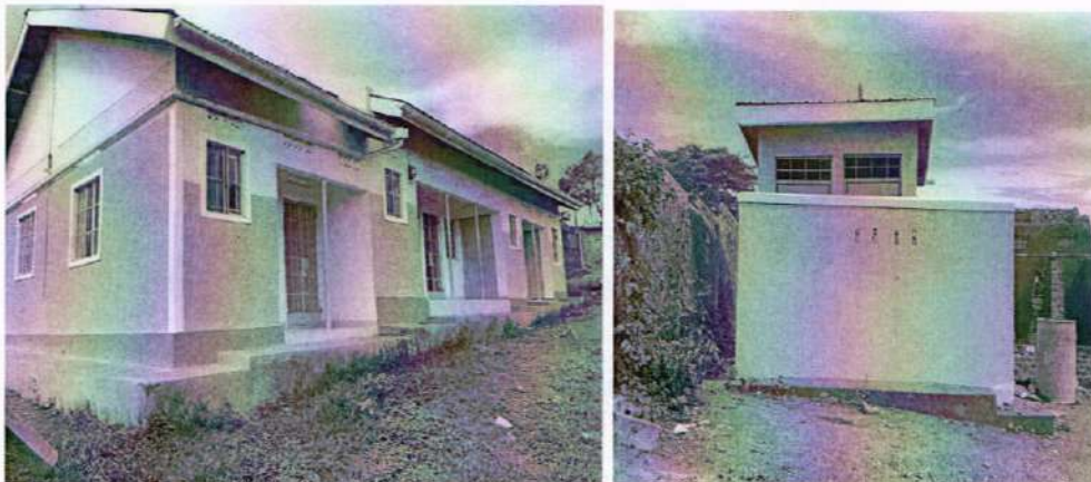
Above: The side view of the renovated staff house and the 2 stance VIP Latrine.
