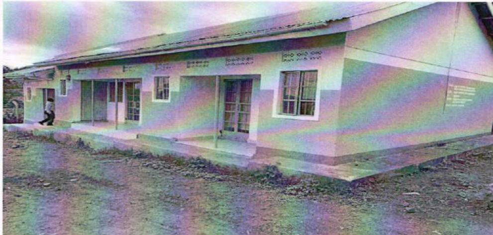
Above: The front view of the renovated staff house showing the extension of another unit.
