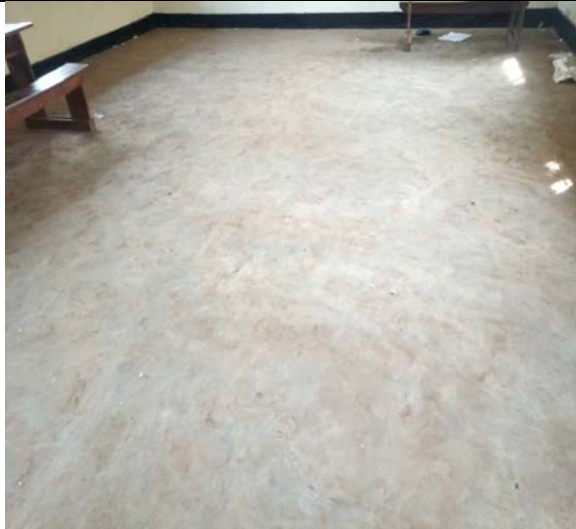
Cracks in the floor area at Mayor Mbale Primary School were rectified.
