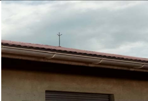
Lightening arrester at 3 class room block at Mayor Mbale Primary School fixed.
