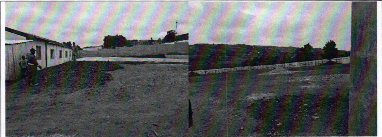
Campsite under construction as at 12 th June 2025 with the laboratories and equipment not yet in place
