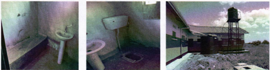
Missing toilet accessories including shower heads, toilet roll holders, soap dishes, PWDs hinged support grabrails; and incomplete water system including missing manholes, gully traps, soak pits, and septic tanks, respectively.
