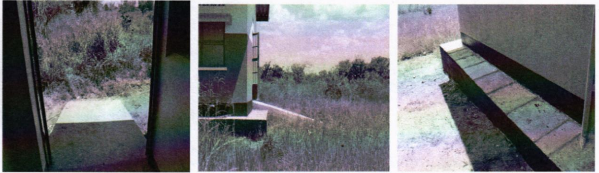
Inaccessible ramp, bushy site and poorly cast splash apron respectively
