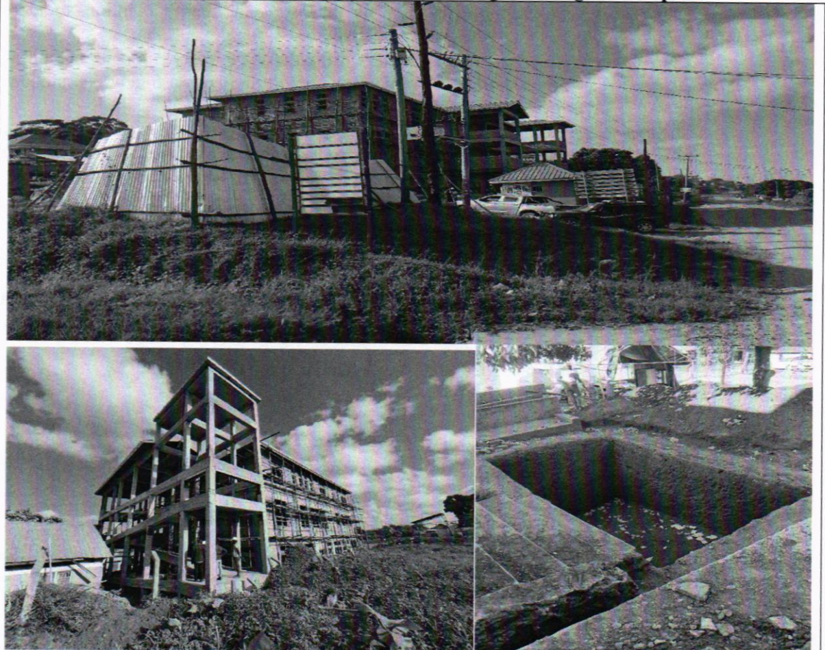
Figure 3: Site not hoarded off with only traces of existing hoardings at first phase
